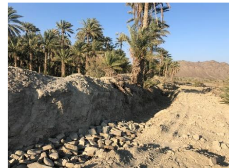
Figure 5. Flood Protection Wall Initiated by PHED Department on Eastern Side of the Chapkol River
